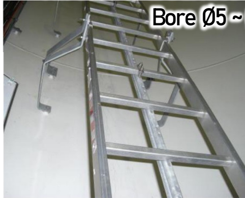
Ladder in Wind Turbine Tower
