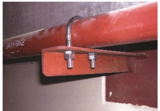
Piping in Power Plant
